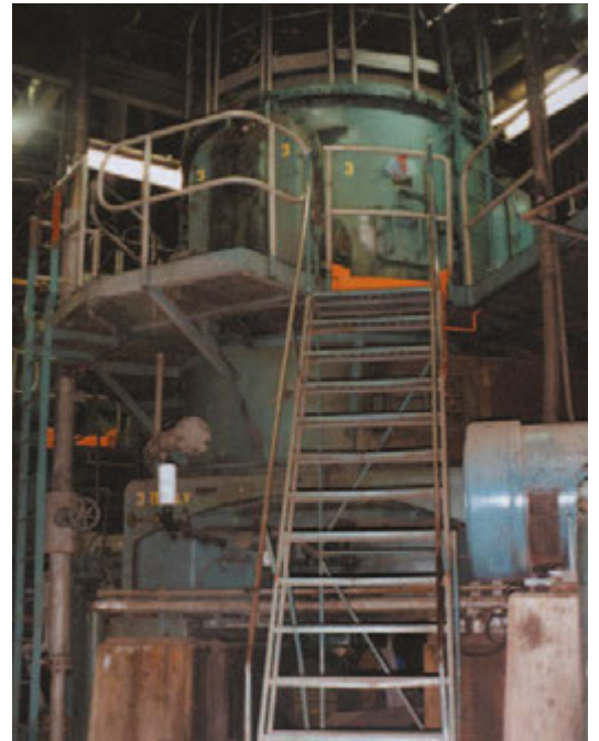
Combustion Engineering 783RP Bowl-Mill Coal Pulverizer.
