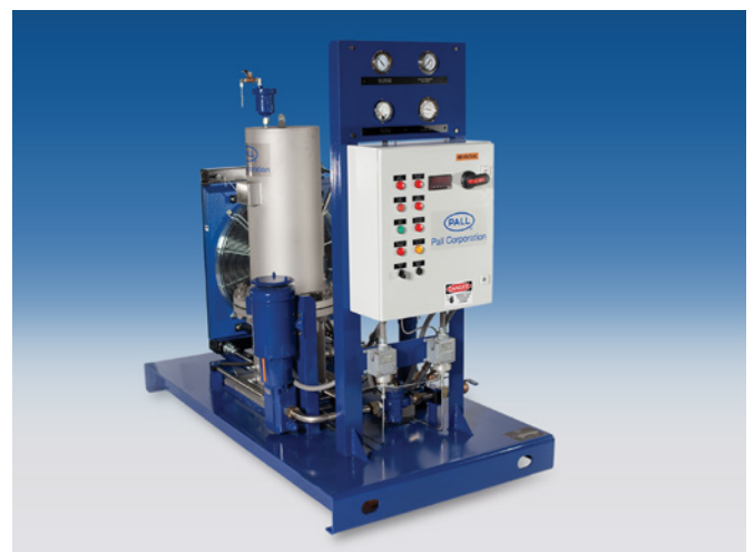
This Varnish Removal Filter skid was used to treat two operating turbines.
